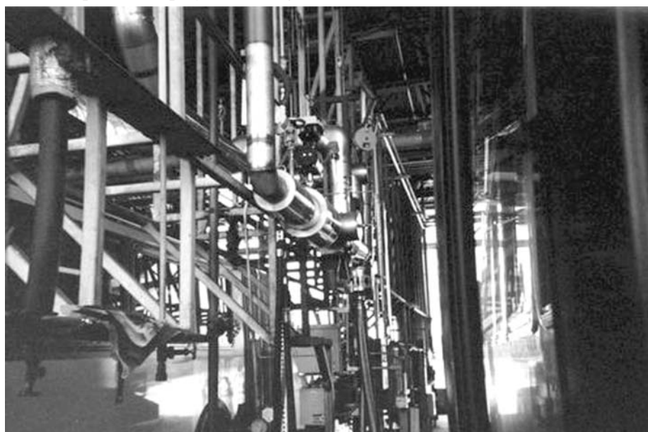
LNG fuel lines inside fueling bay, Dallas Area Rapid Transit (DART)
