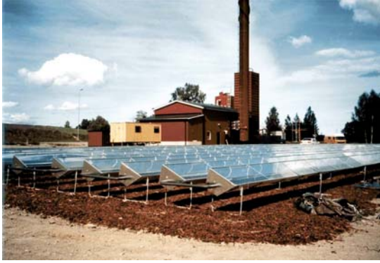
Fig. 32 A field of 500m 2 stand-alone MaReCo collectors constructed 1999 in front of the bio fuel burner in Torsåker, Sweden. Each collector has a length of 40 meter.
